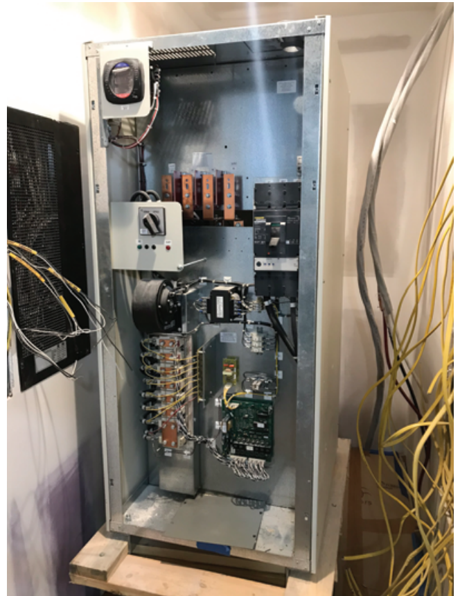
Custom-made isolation transformer.
