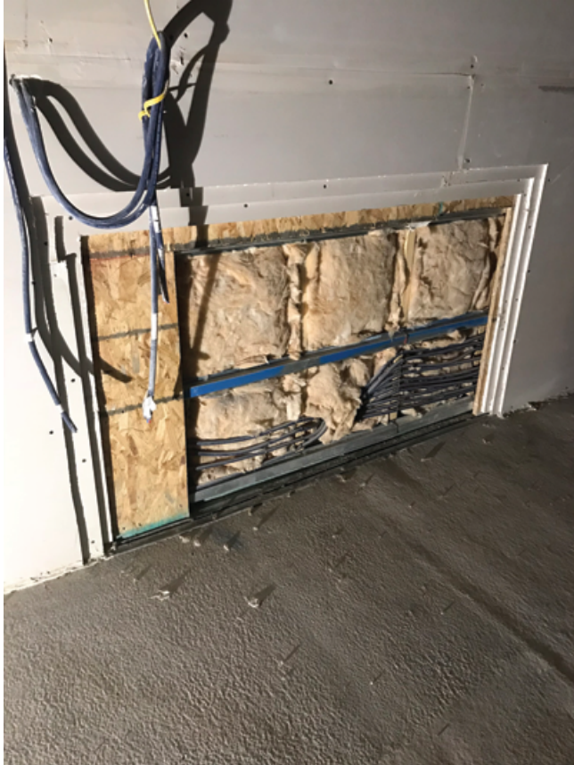
The floating floor is made up of nine inches of concrete, sandwiching acoustic isolation pads.
